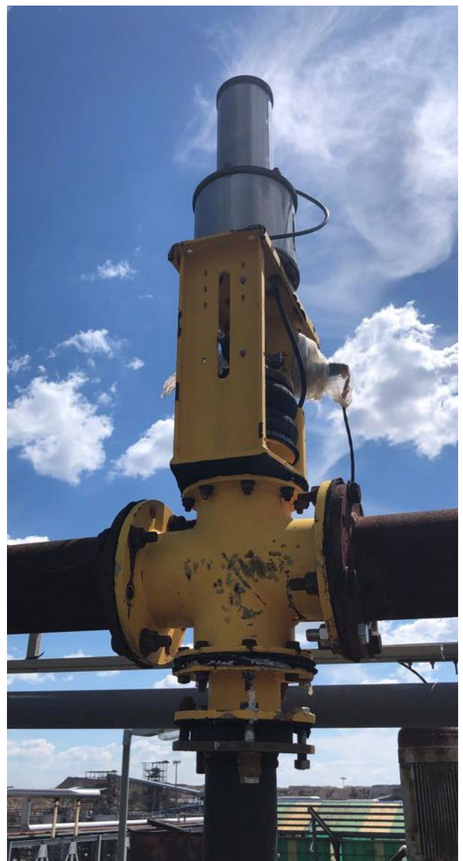
Dosing valve on the lime ring main
